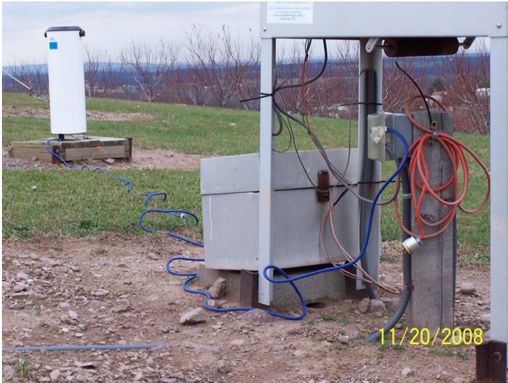
Figure 5-2. Power Cords Not Secure and Gage Not Level
