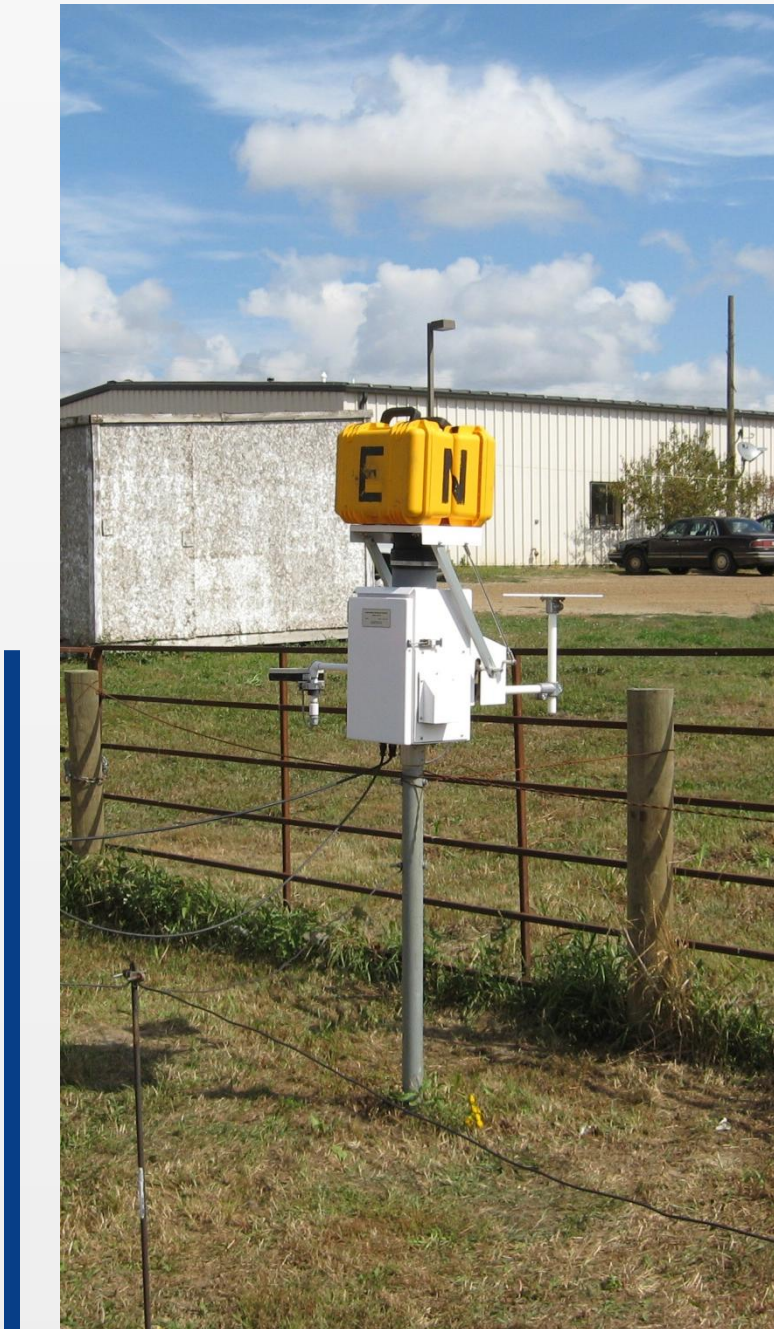
March 2007 first MDN N-CON installed at SD18
