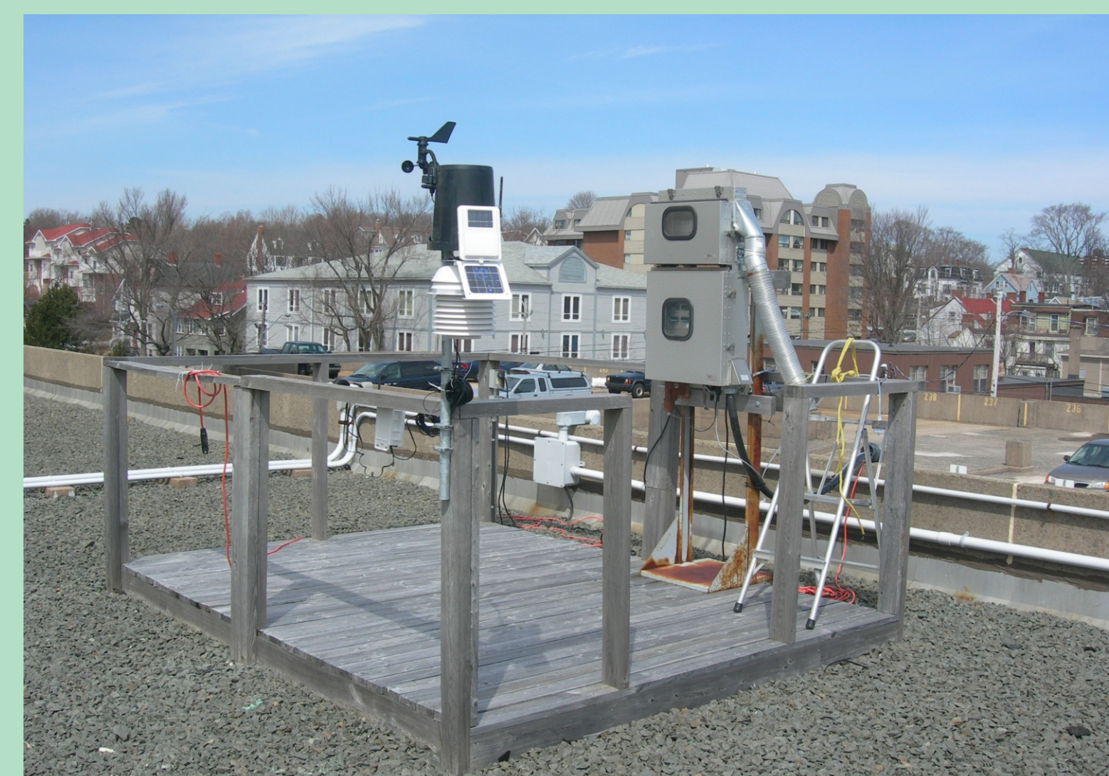
Illustration of the Tekran sampling apparatus and Davis weather system on the roof deck.
